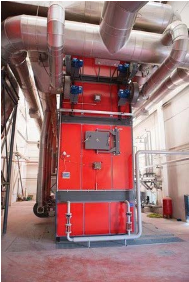
Grouping use of a biomass boiler to substitute the fossil fuel.
